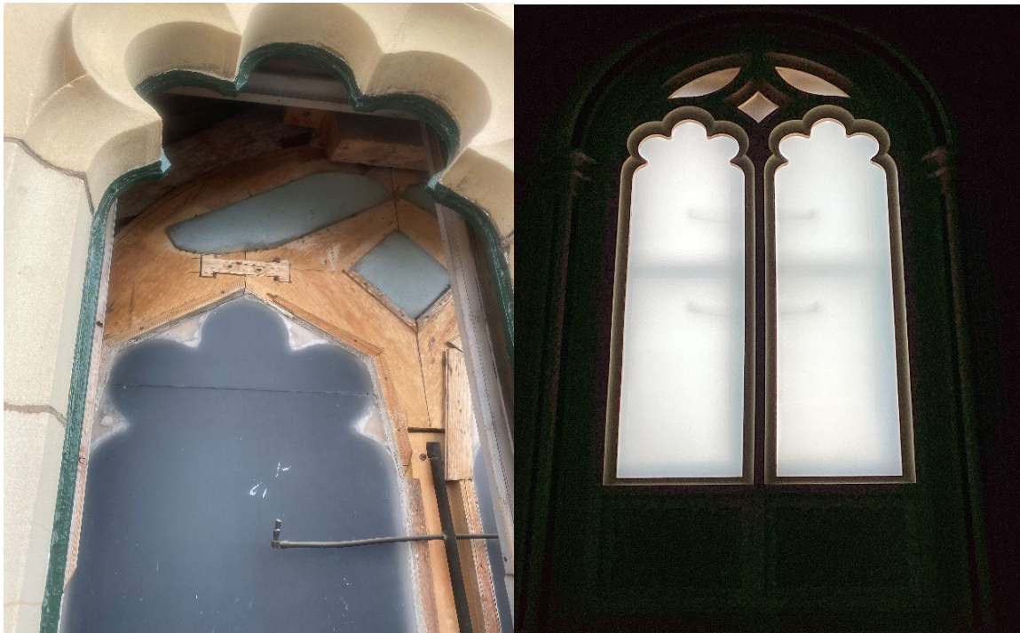
Original glass from within the cavity and the new laminated glass installed as viewed from inside the Ball Room
